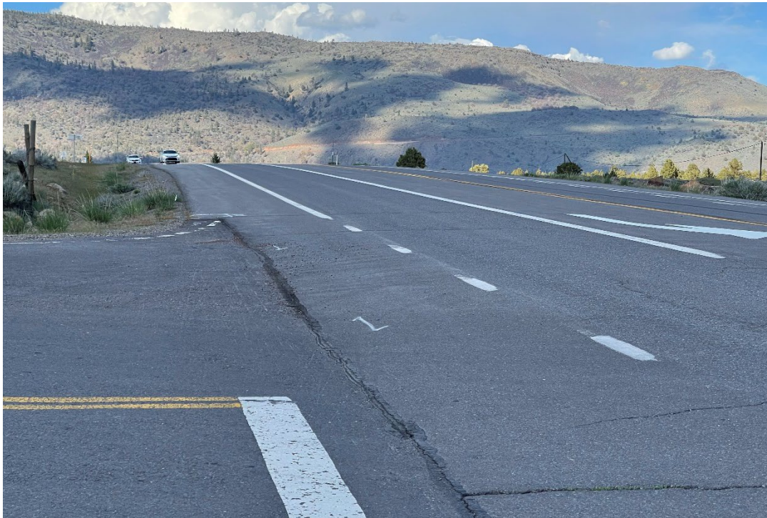
Figure 4-6: Limited Sight Distance at Spring Ridge Drive Intersection
